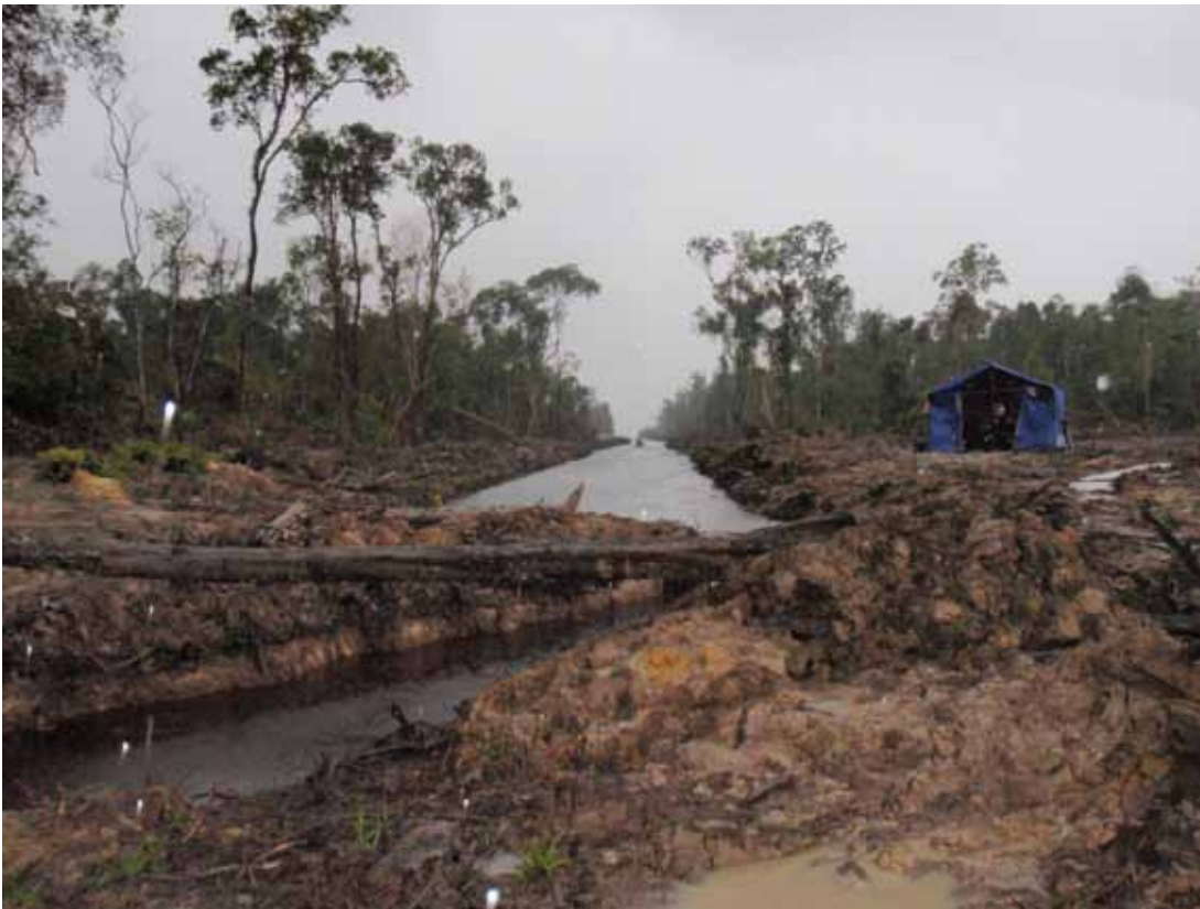
Image 12. One of the canals constructed in PT Bumi Sawit Sejahtera. This development is located in Conversion Forest.
