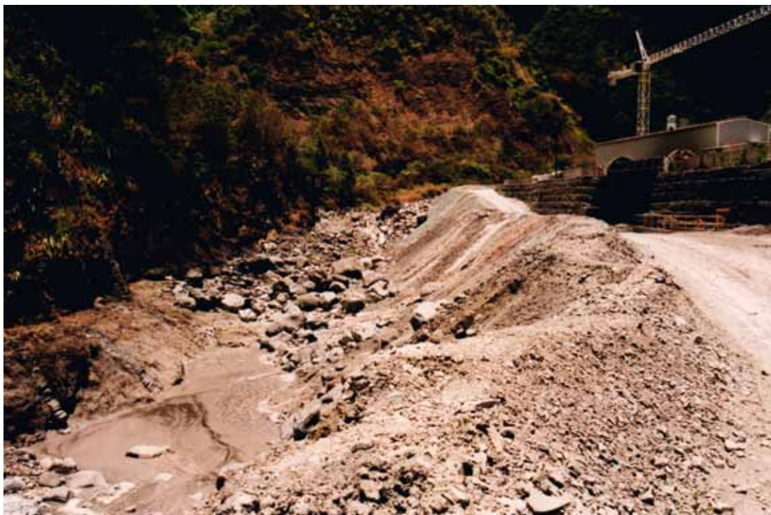
Figure 23 – Hydraulic project causing major damage to a major mountain aquifer, threatening coral reef and partially funded by EU structural funds. Reunion Island, French Oversea Region. ©SREPEN, 2006
